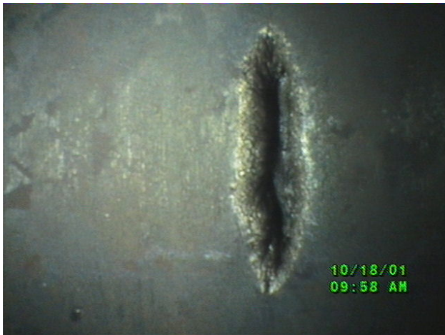
Figure 2. Leak #2 in FWH 81E
