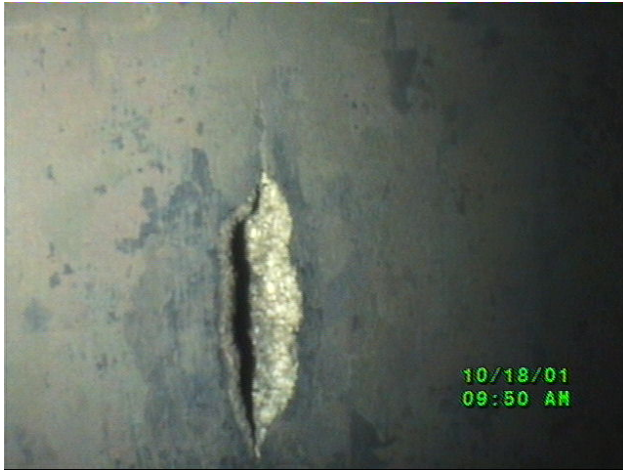
Figure 1. Leak #1 in FWH 81E
