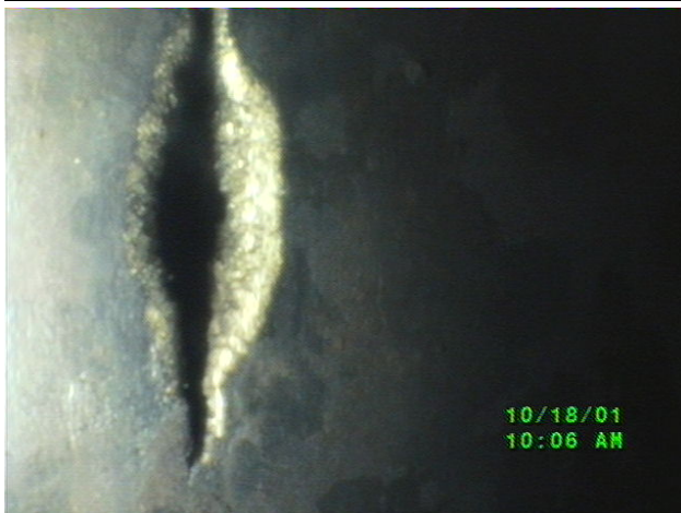
Figure 3. Leak #3 in FWH 81E
